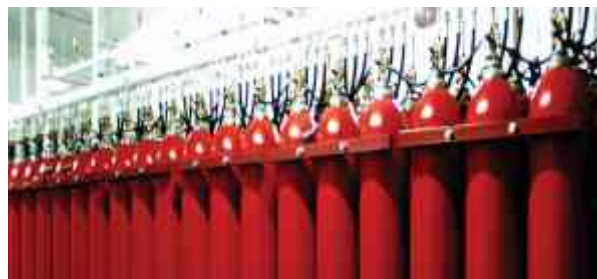
FIRE SUPPRESSION SYSTEMS
