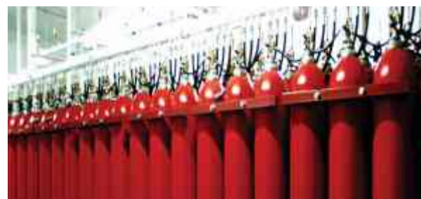
FIRE SUPPRESSION SYSTEMS
