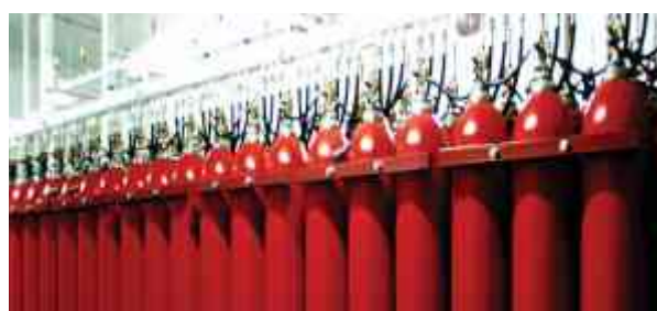
FIRE SUPPRESSION SYSTEMS
