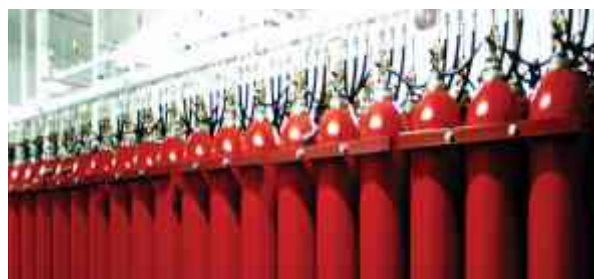
FIRE SUPPRESSION SYSTEMS
